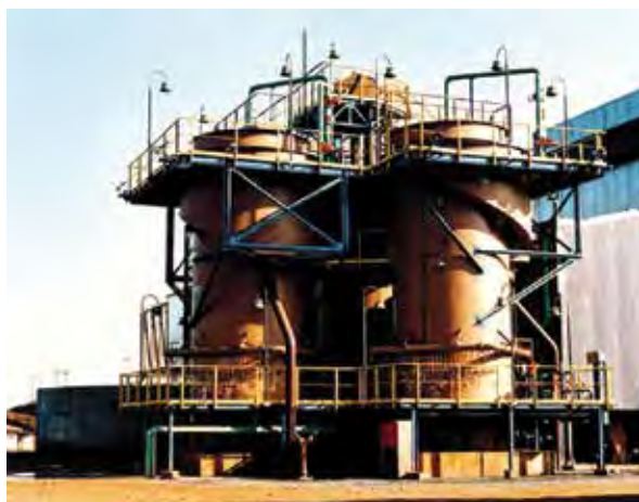
FIGURE 3 Column flotation plants are inexpensive and compact
