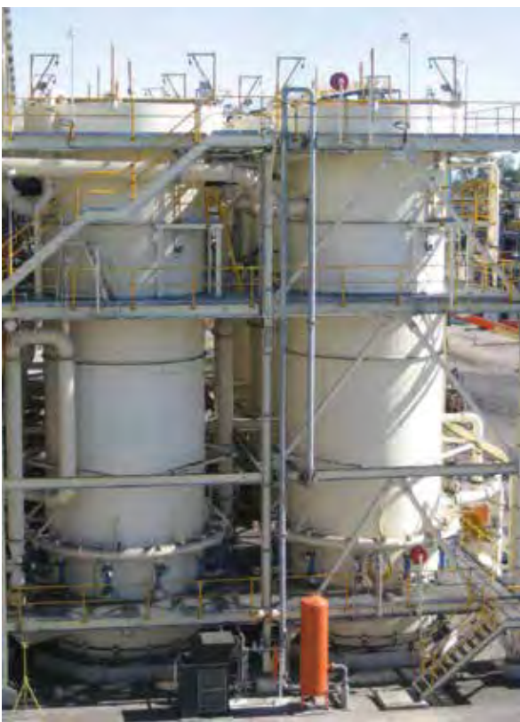
FIGURE 3 Column flotation plants are inexpensive and compact
