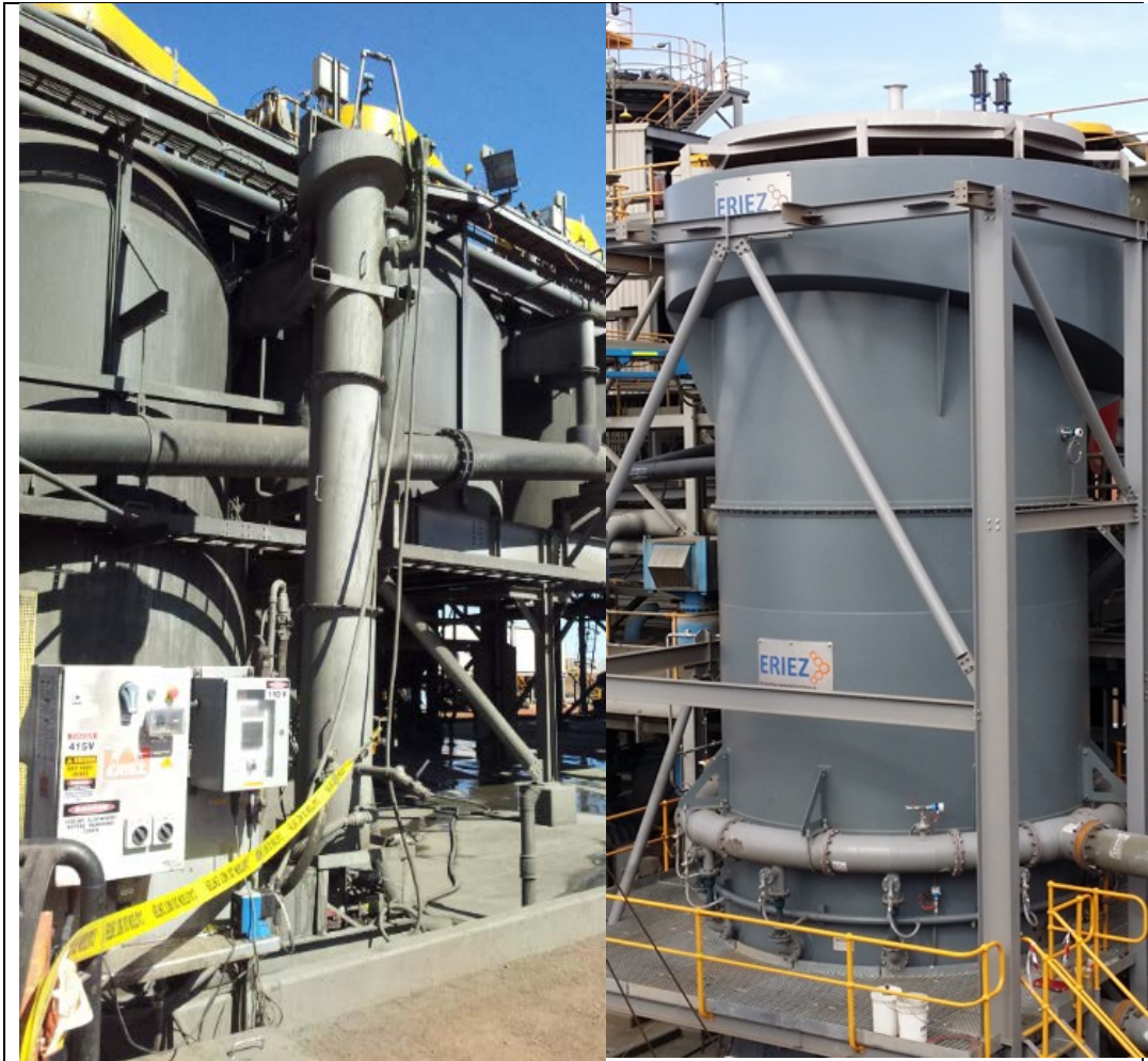
Figure 6: Photograph showing the installation of the industrial column flotation cell and 500mm pilot column unit.
